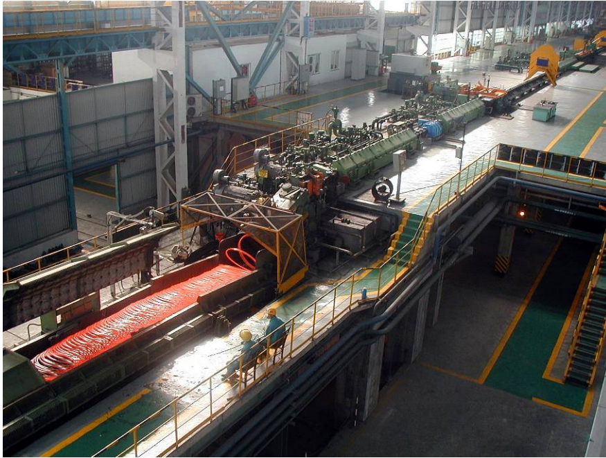
Rod outlet equipped by Siemens.
