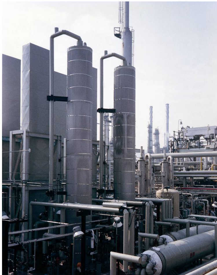
Zimpro wet air oxidation system installed in China.
